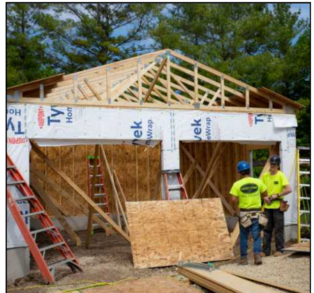
Pictured above: OFS staff and build academy crew members working on garage at MACLT acquisition-rehabilitation project. Pictured left: Front of home after was complete by OFS staff and build academy crew.
